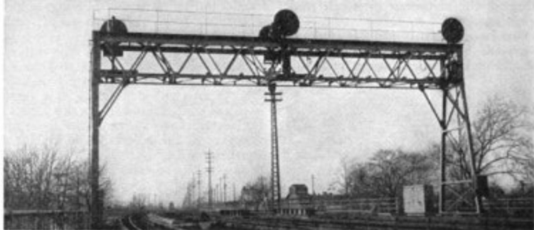
Westward home-signal bridge showing flashing-light train-order signal mounted between the top and bottom arms of each signal
