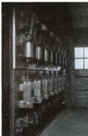
Interior of third-rail breaker house showing remote controlled circuit breaker
