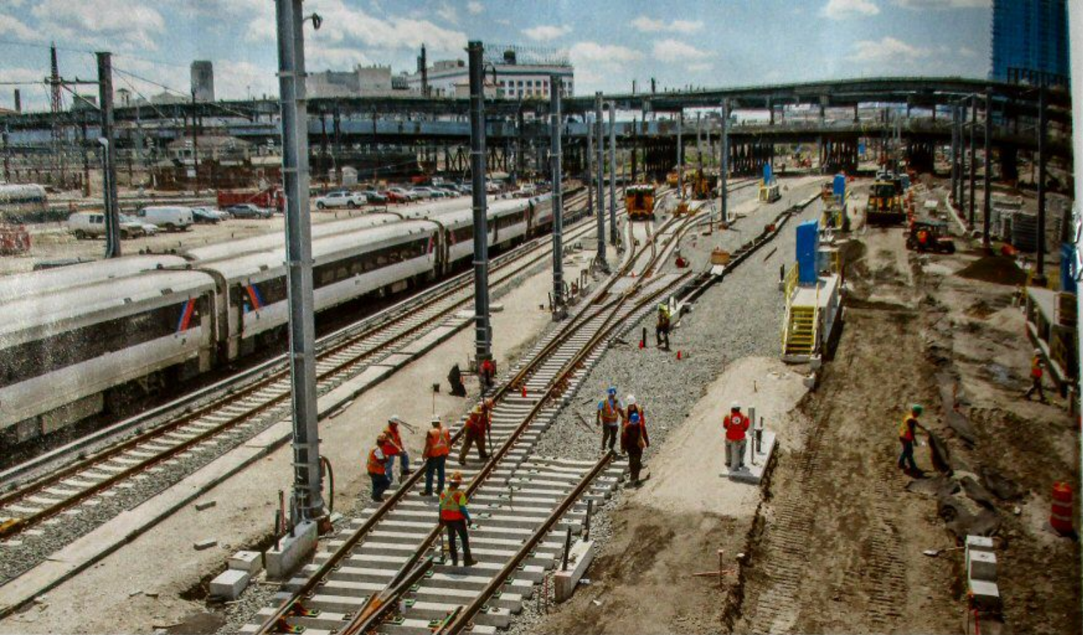
Construction crews install track at the Mid-Day Storage Yard in Long Island City, Queens. Located on the site of the former LIRR Yard A, adjacent to Northern Boulevard, trains will reach it via a tunnel that branches off from the Manhattan tunnels.
