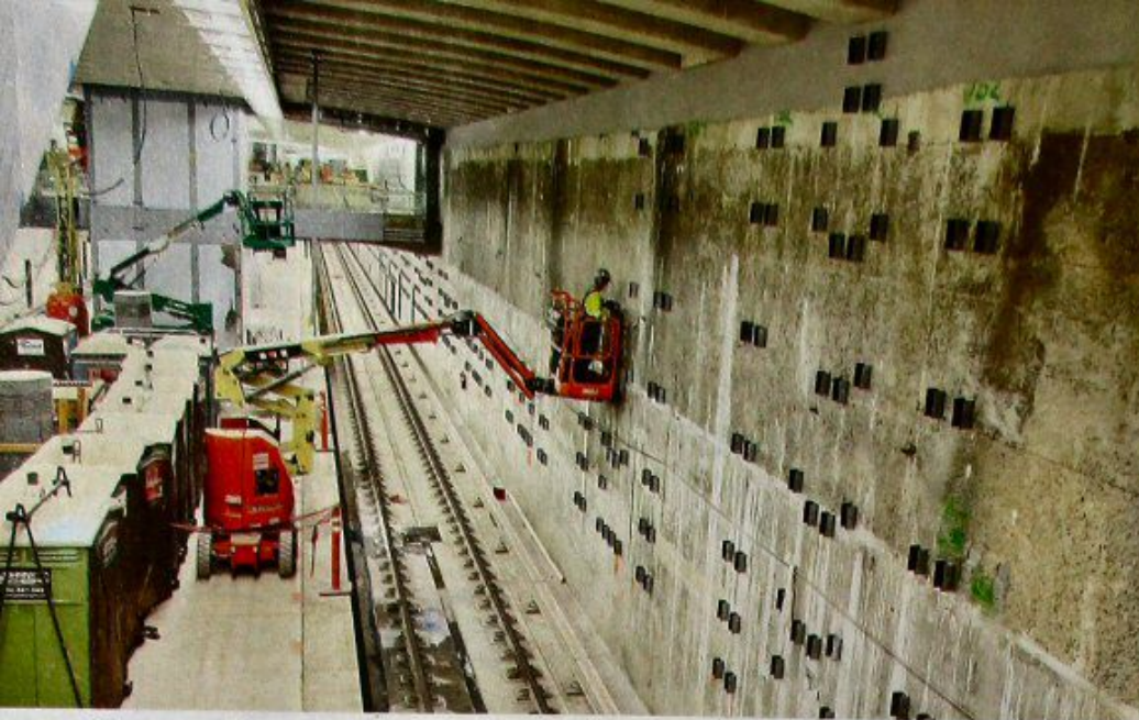
The caverns housing the new terminal below Grand Central are 1,143 feet long. For six years, 1,000 employees working 24 hours a day, five days a week blasted out the new spaces.
