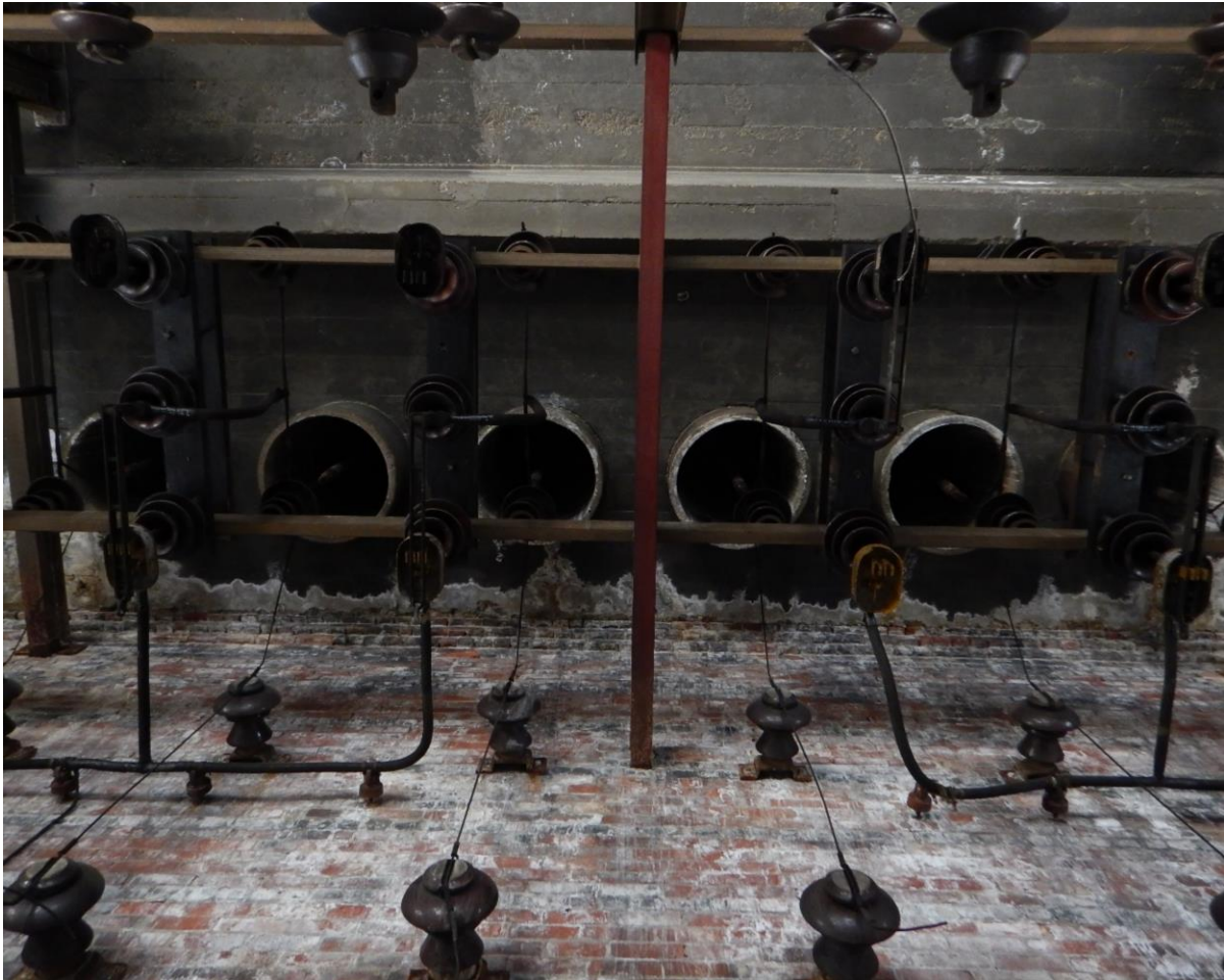
PHOTO 40. EXTANT SUBSTATION EQUIPMENT PROTRUDING THROUGH ROOF
