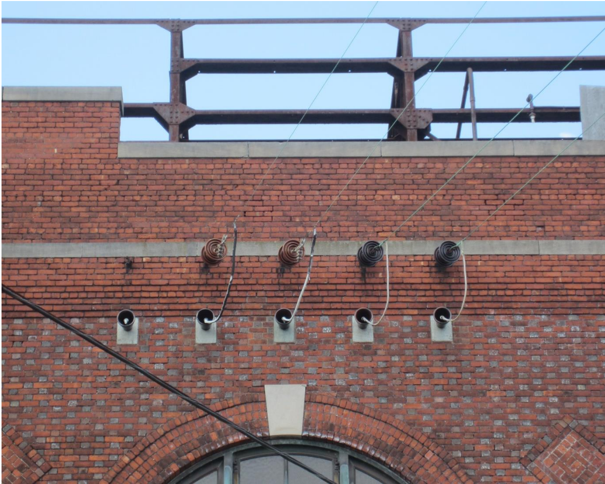
PHOTO 05. EAST ELEVATION EXTANT SUBSTATION EQUIPMENT
