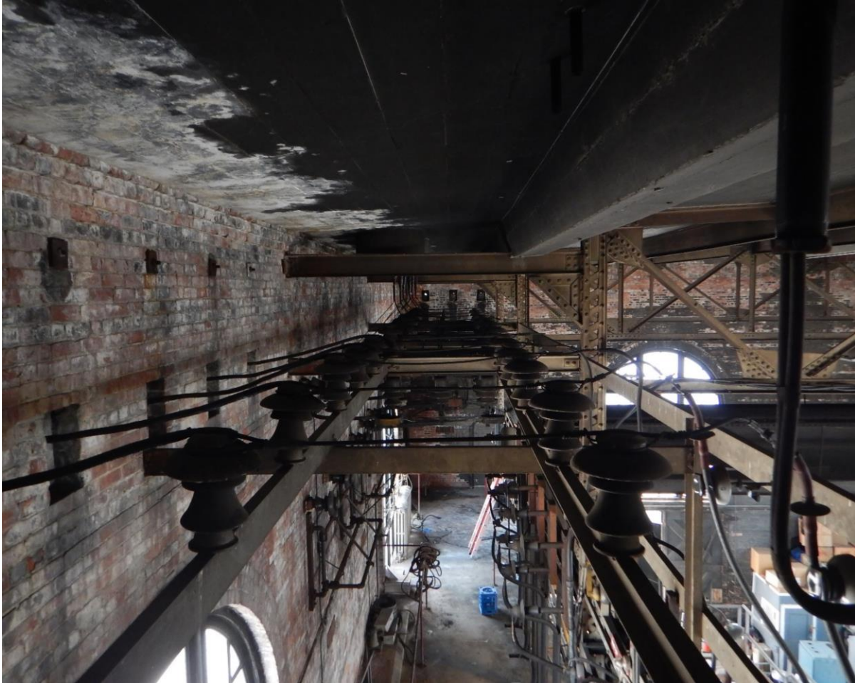
PHOTO 49. EXTANT SUBSTATION EQUIPMENT
