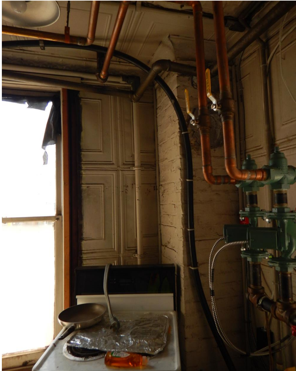
PHOTO 73. FIRST FLOOR MECHANICAL ROOM FACING EAST
