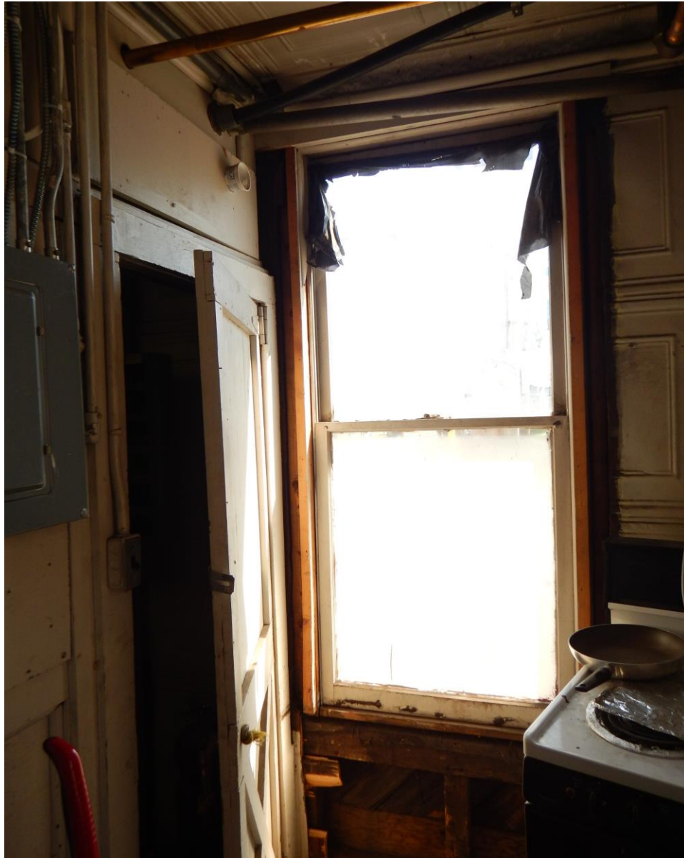
PHOTO 74. FIRST FLOOR MECHANICAL ROOM FACING EAST
