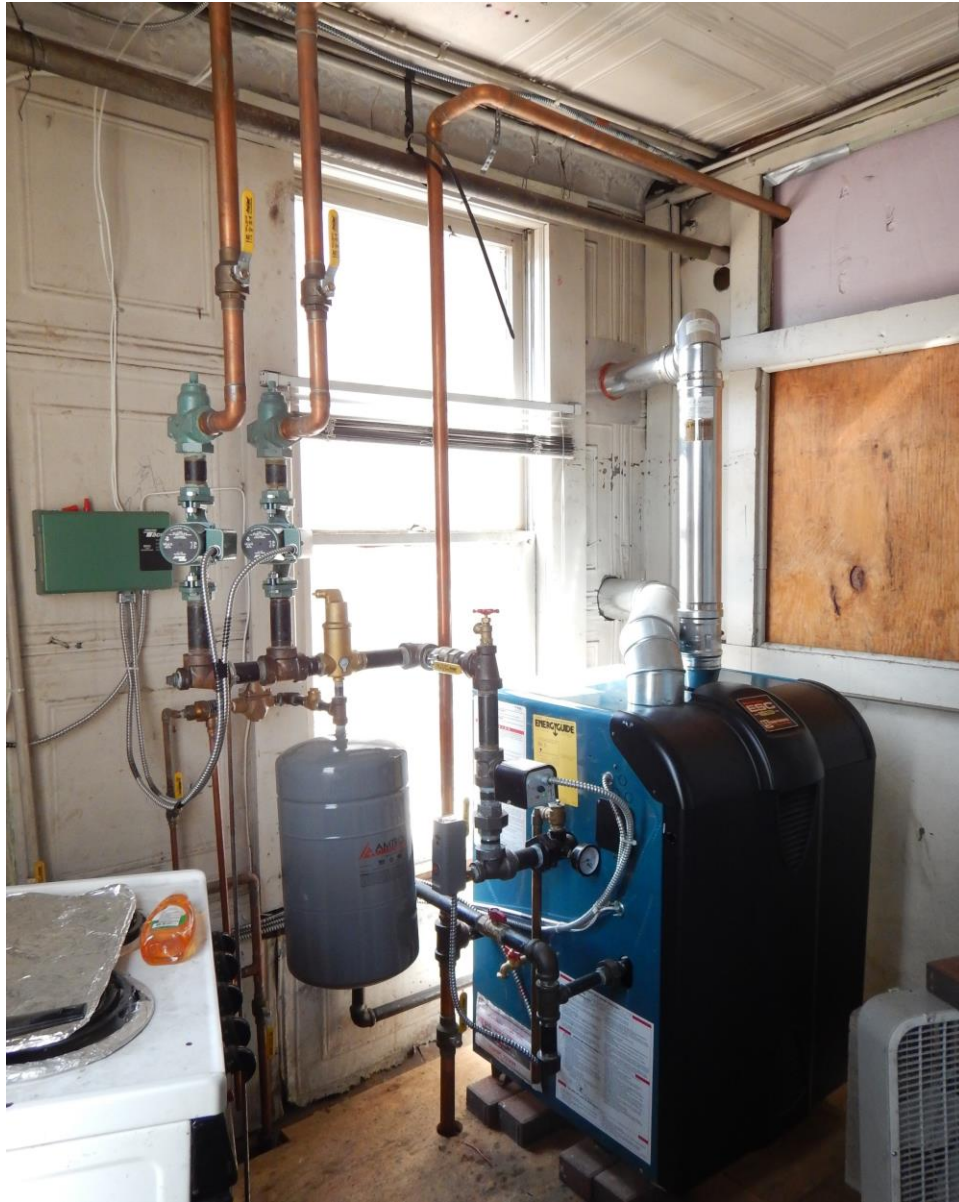
PHOTO 72. FIRST FLOOR MECHANICAL ROOM FACING SOUTHWEST
