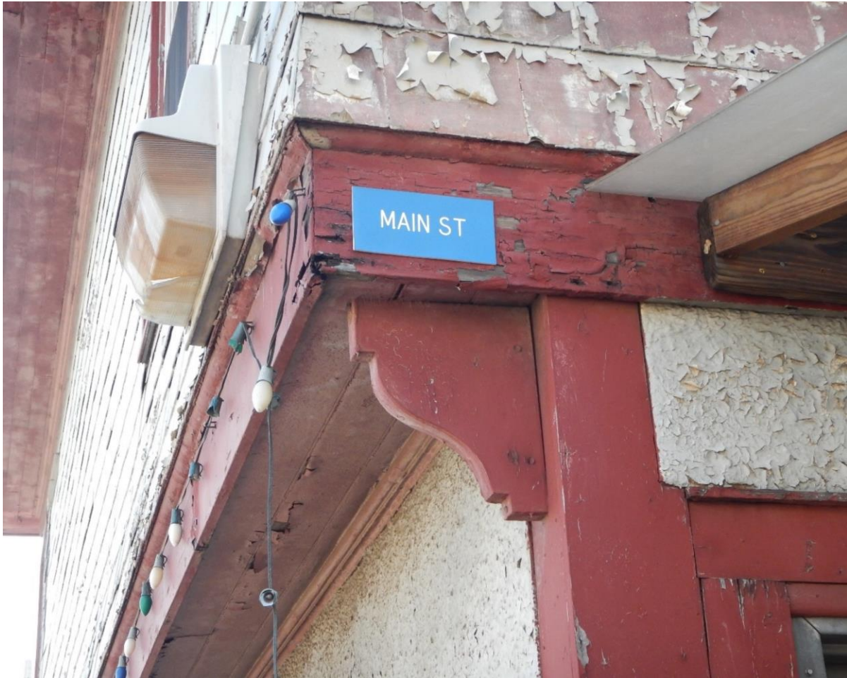
PHOTO 63. NORTHWEST WOOD BRACKET DETAIL
