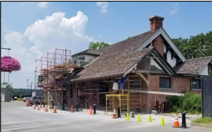
The historic Oyster Bay Train Station is in the final stages of exterior restoration work on south and west sides.
