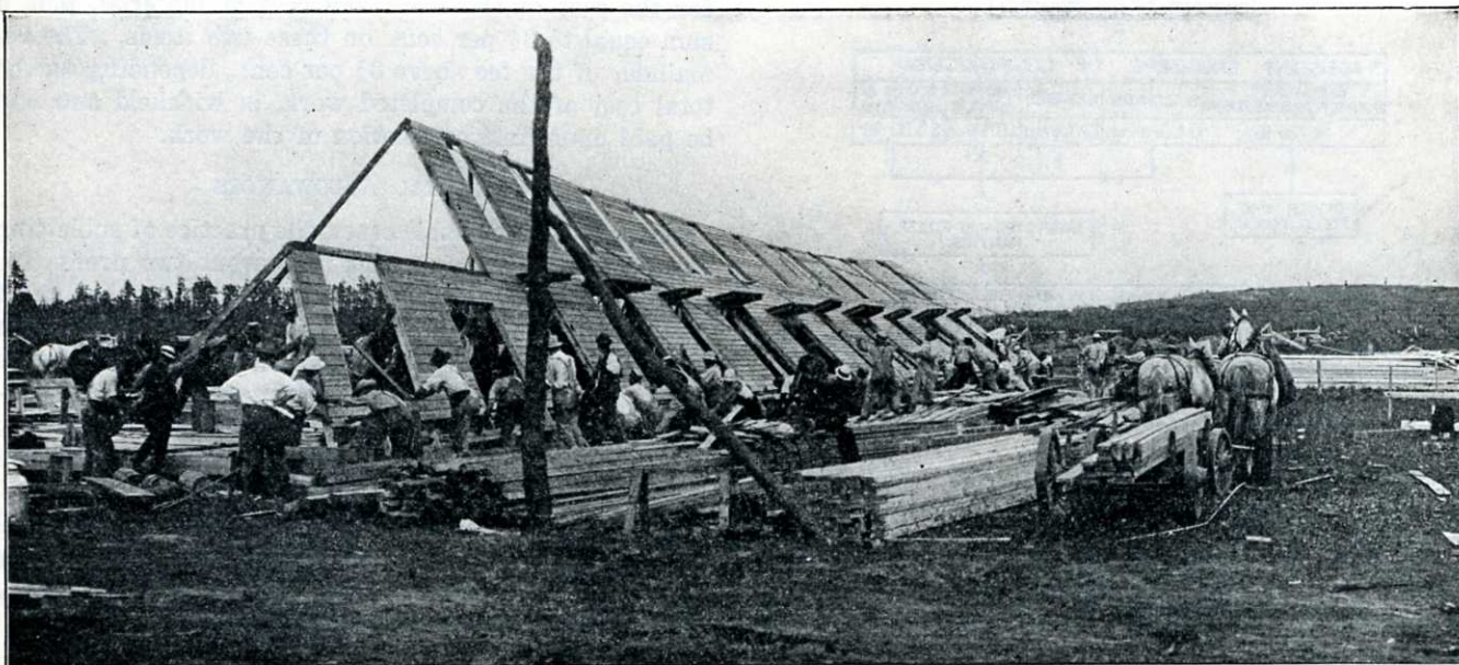
ALL HANDS RAISE THE FINISHED WALL INTO A VERTICAL POSITION—THIS SCHEME OF CONSTRUCTION ELIMINATES ALL SCAFFOLDING
